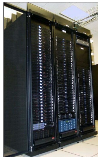
Pictured above: The Bioinformatics Cluster is housed in a dedicated computing facility that provides battery backed up power, tape backups, independent airconditioning and 24/7 on site personnel. It is connected to the campus backbone, thus ensuring a 1GB link to every desktop of the new offices of the Center for Bioinformatics.
